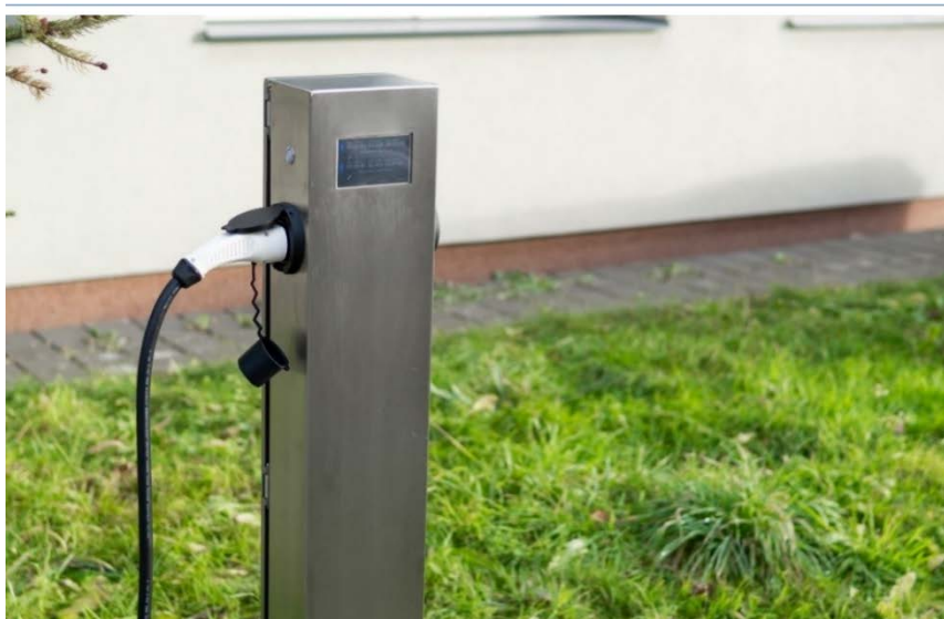
Figure 6: Example of a charging column for two BEVs with a power output of 22 kW
